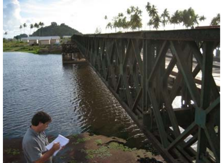
Man at work: Dave takes notes at one of the road's 42 existing bridges
